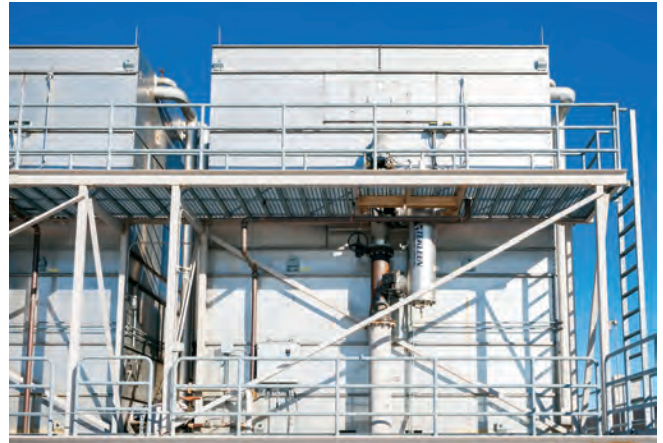
Back side of cooling towers at terminal 2, showing one of the two installed Tekleen filters. It is the large cylinder hanging vertically beneath the walkway.
