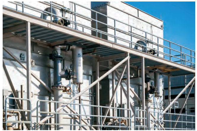
Back side of cooling towers at terminal 2, showing both Tekleen filters.
