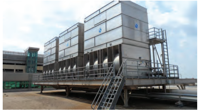
Front side of cooling towers at terminal 2 (Humphrey Terminal)
